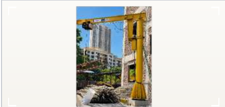
05 Jib Cranes Wall & pillar-mounted jib cranes for workstations and machine cells.
