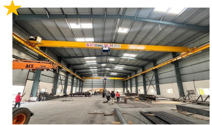
Single Girder EOT Crane
